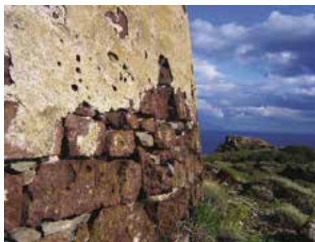
Figure 9 – Tower of Zenòbito: the eroded masonry with the ancient plaster
