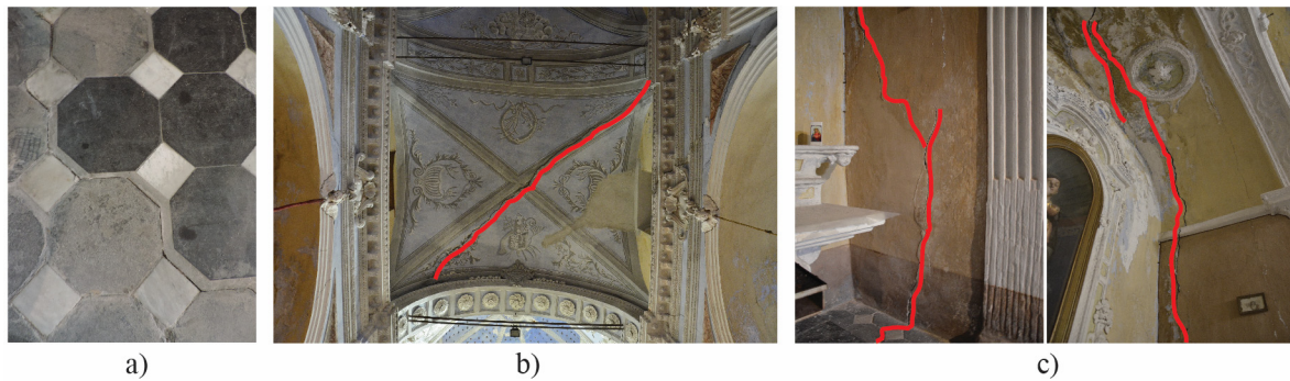
Figure 9: Damage observed in Santa Margherita church in Diano Arentino: a) large gap in the floor, b) diagonal shear cracks of vaults, c) vertical crack progressing over the entire height of the wall from floor to vaults.
