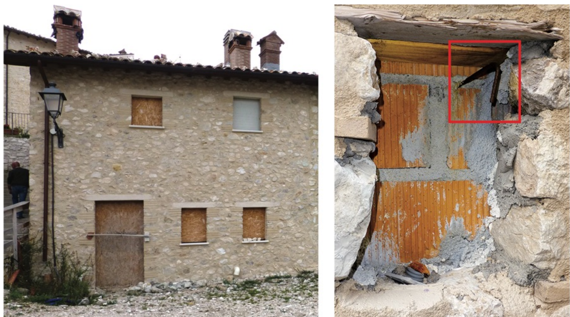
Fig. 18. Demolished and rebuilt clay block masonry with connected natural stone veneer. Norcia, Castelluccio di Norcia. a) General view, b) close up of a cavity, with clay block and connection rebar visible within the red frame.
