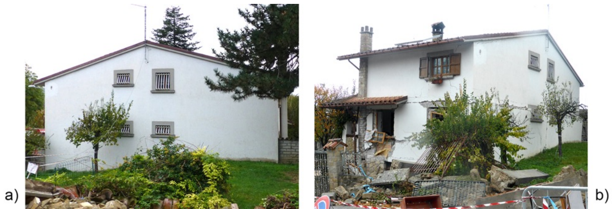
Fig. 21. Solid concrete block masonry building. a) After the 24 th August event, b) after the 30 th October event. Amatrice, viale Saturnino Muzii.
