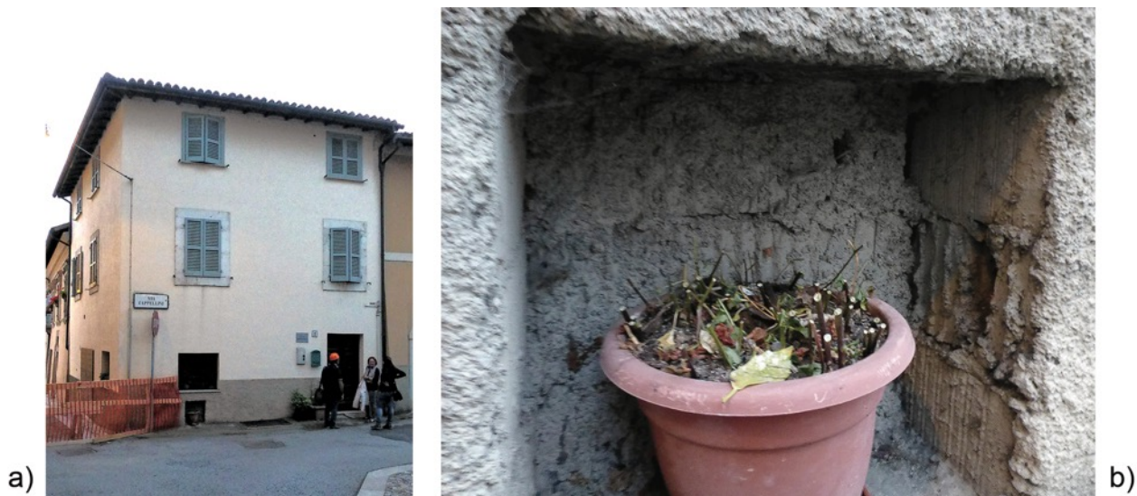
Fig. 19. Demolished and rebuilt plastered clay block masonry. a) General view, b) close up of a cavity, with clay block visible. Norcia, via Anicia intersection with via Cappellini.
