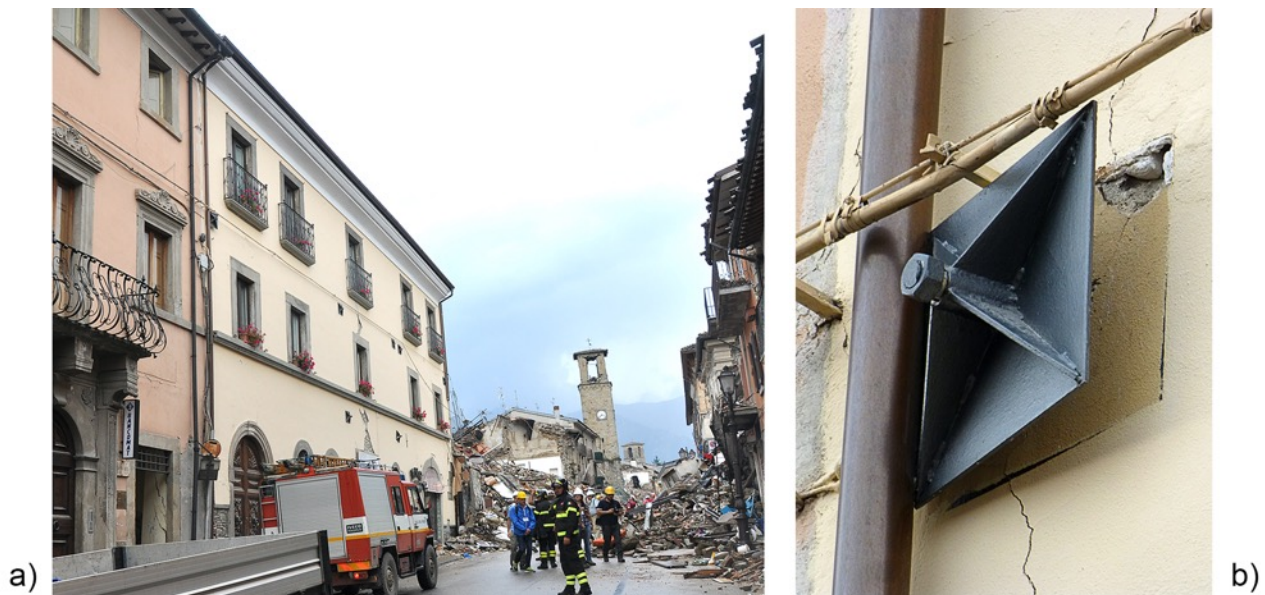
Fig. 8. Steel tie rods in the lightly coloured building, Amatrice, corso Umberto I. a) General view; b) Close up of a wall anchor.
