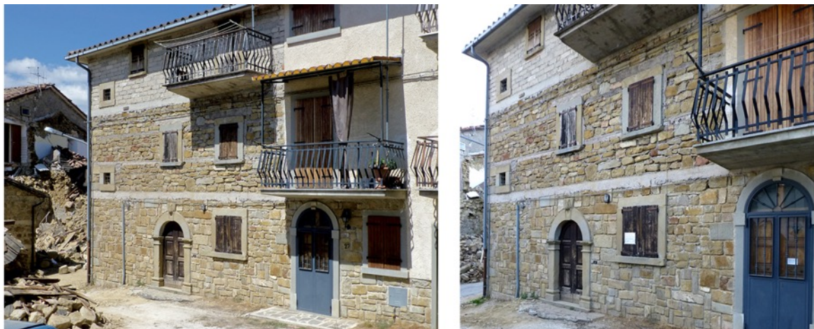
Fig. 17. Demolished and rebuilt natural stone masonry, resorting to modern mortar and ring beams. Amatrice, San Capone. a) Post 24 th August; b) Post 30 th October.
