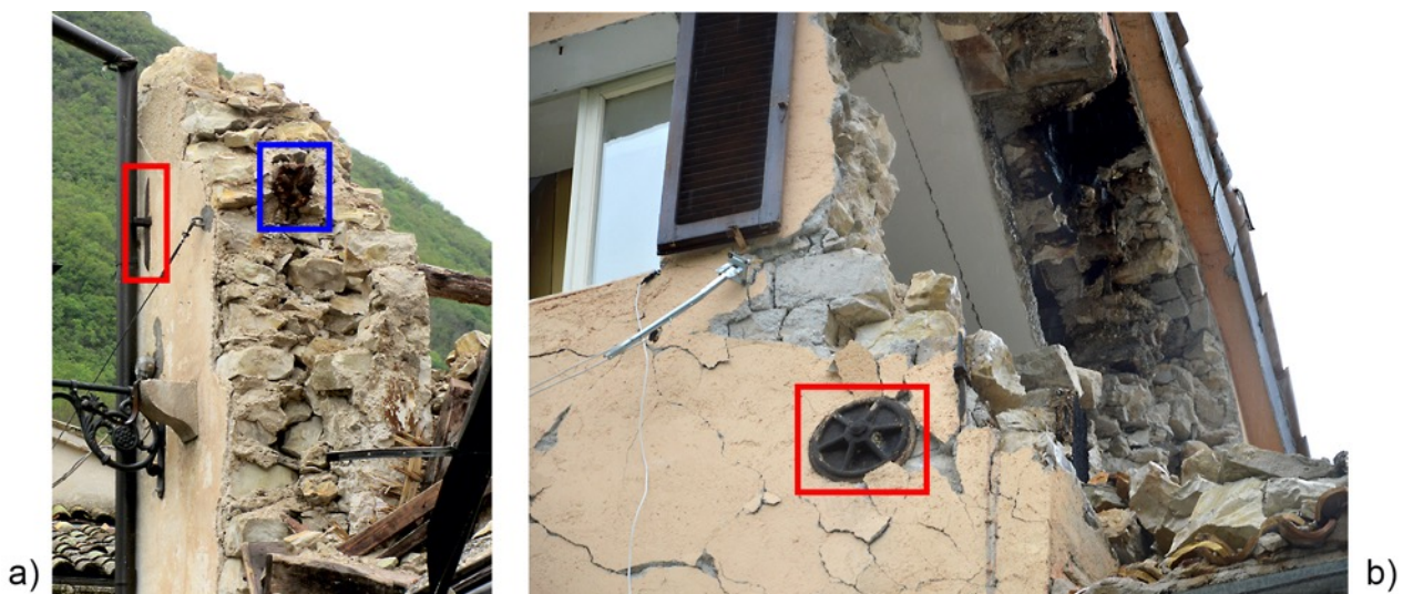
Fig. 4. Timber tie rods (blue frame) and steel wall anchors (red frame) in Castelsantangelo s/N: a) Via Parco della Rimmembranza, b) via delle Mura Castellane.
