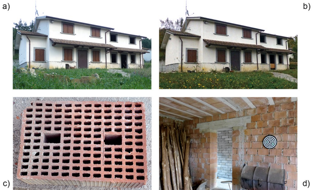
Fig. 20. Clay block masonry building. a) After the 24 th August event, b) after the 30 th October event, c) close up of a block, d) view of bare wall and floor. Amatrice, San Capone.
