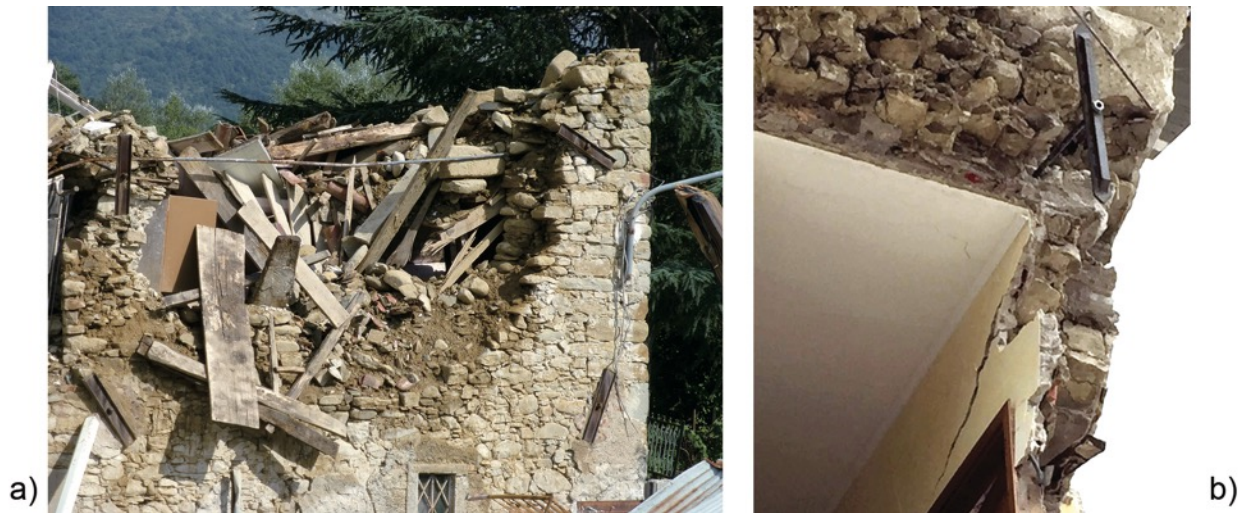
Fig. 13. Collapse of a masonry building having steel ties combined to poor mortar. a) Amatrice, Petrana; b) Arquata d/T, Piazza Umberto I.
