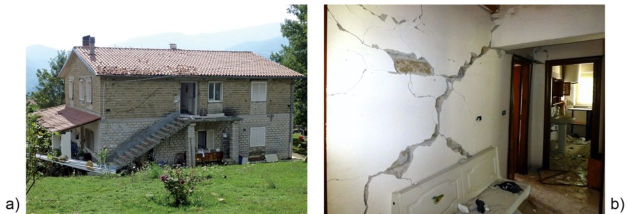
Fig. 22. Solid concrete block masonry (ground floor) and tuff masonry (first floor) building. a) External view, b) Internal view at first floor above ground. Accumoli, Illica.
