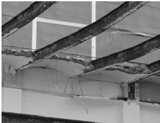
Figure 10. Details of a floor system observed during the demolition of an Eixample building.
