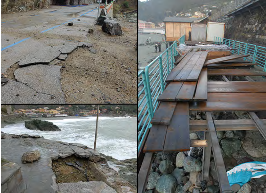
Figure 15: Damage to promenade and touristic structures after 2008 storm surge
