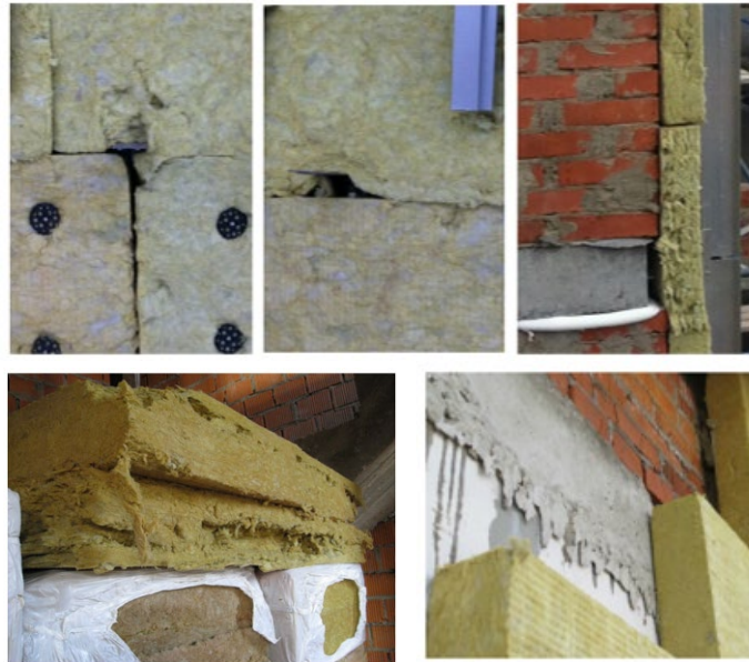
Figure 1. Defects in thermal protection: from top to bottom and from left to right: gap at the junction of the insulation boards; gap at the junction of the bracket with insulation; detachment of the insulation from the foundation; defects in materials; level defects.
