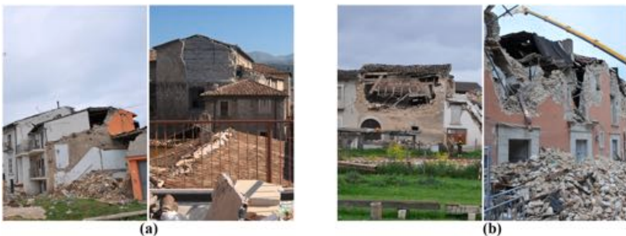
Fig. 3. Typical OOP failure mechanisms in the 2009 L’Aquila earthquake with collapses of (a) gables and (b) main façades. Photo courtesy of Simone Del Grosso.
