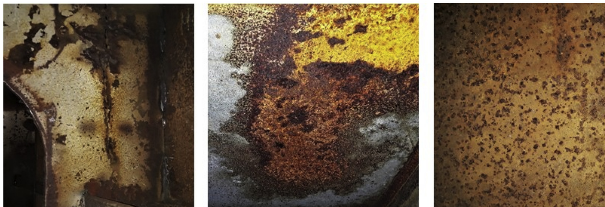
Fig. 5. From the left: example of crack, corrosion and pitting occurring in the testing facility structures.
