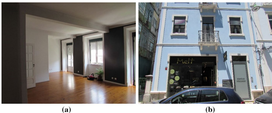
Fig. 3 Alterations: a removal of internal walls to have larger rooms and b removal of masonry piers to have large shop window
