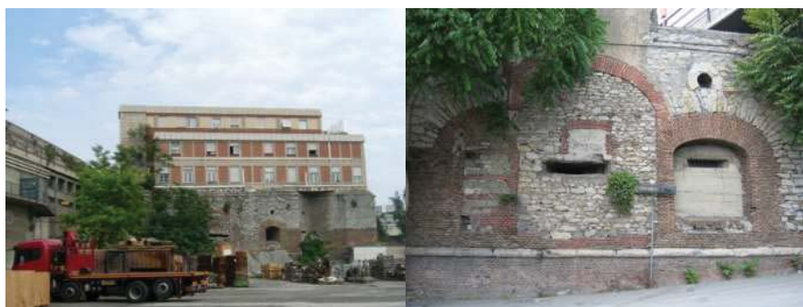
Figg.10a, b : The Battery today: western elevation (a) and detail of the eastern elevation (b), subject to the stratigraphic analysis. Above the cannon embrasure a circular opening can be seen for dissipating the gun smoke
