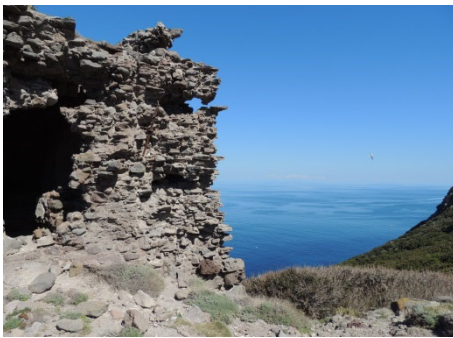
Fig.7 - Tower of Barbici: the deeply eroded masonry.
