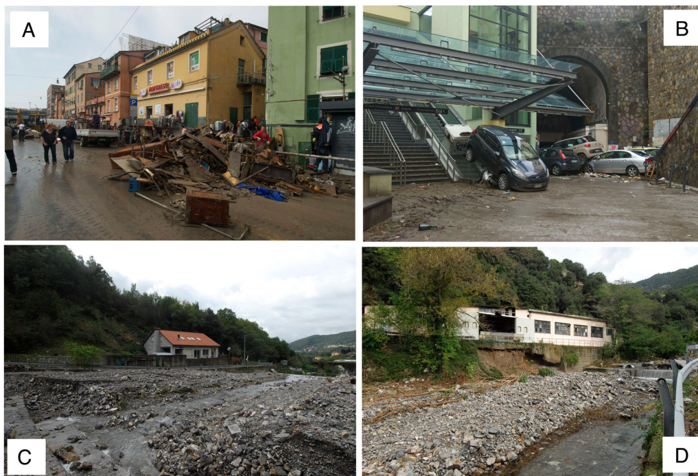
Figure 5. Damage after 2014 flood in the Bisagno catchment; A, B near the train station; C, D solid transport and riverbank collapse along Geirato stream, a Bisagno river tributary (refer to the scheme in the Main Map).
