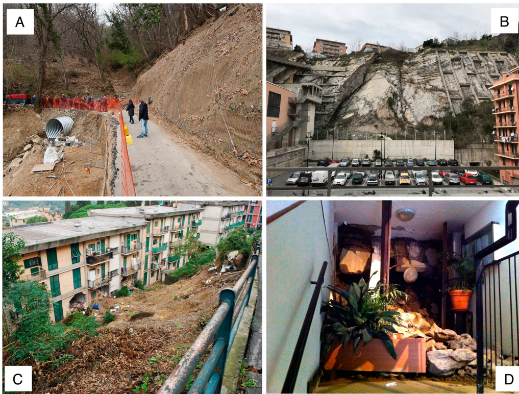
Figure 6. Landslides in the Municipality: A, road interruption in the upper Urban unit 12; B the actual status of the via Digione collapse landslide (u.u. 27); C landslide affecting a residential building and a road; D of a landslide strongly affected apartment in 2014 (district 15).
