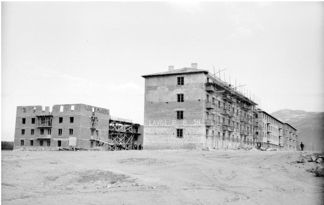
Figure 2. The first housing block (lagje nr. 1) under construction in the new town of Kukës. The graffitied words “Lavdi P.P.SH.” on the wall means “Glory to the Albanian Labour Party”; P.P.SH is the acronym of “Partia e Punës e Shqipërisë” (Courtesy of Arkivi Qendror Teknik i Ndertimit, AQTN, Fototeka, v. 1964).
