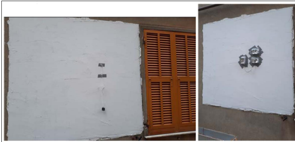
Figure 14. HFM installation to measure the contribution of the nanotechnological mortar. Particular of the external side.
