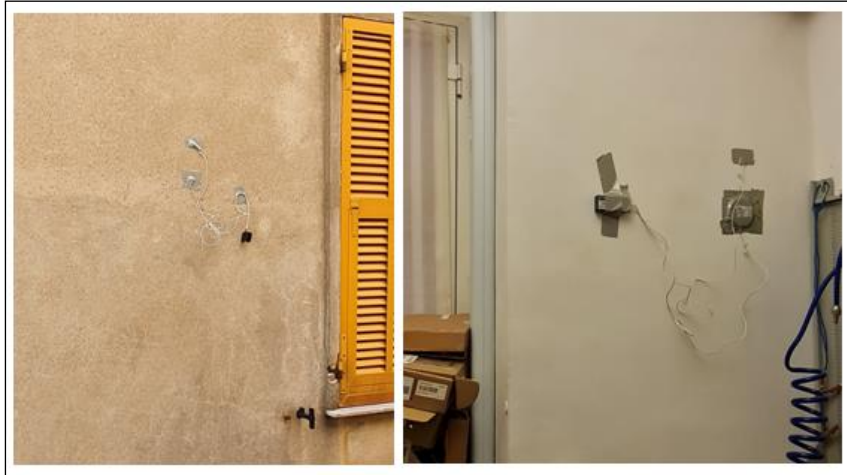
Figure 8. HFM installation on the external (on the left) and internal (on the right) sides.
