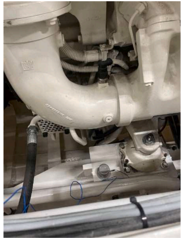
Fig. 1. Resilient mounts used to uncouple the diesel engine from the ship hull, with a mono-axial accelerometer used to measure the vertical vibration levels at the diesel foundation.
