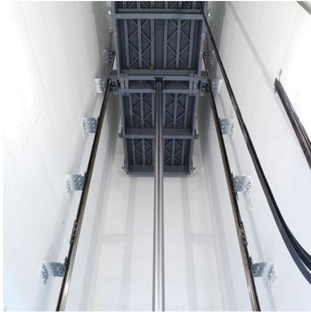
Figure 2.3: A direct hydraulic elevator - note that the weight of the cabin is imposed directly on the piston
